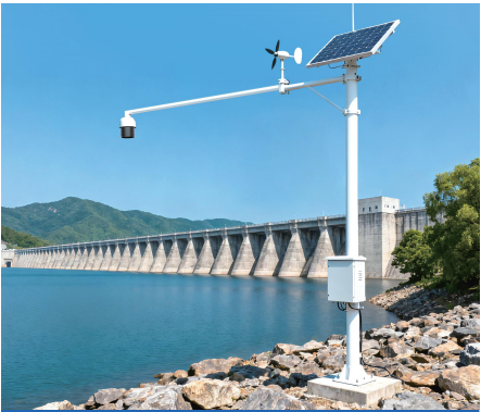
Dam Water Level Monitoring
