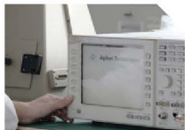
Communication Inspection Equipment
